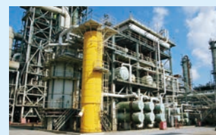
Naphtha Hydrotreating Unit
