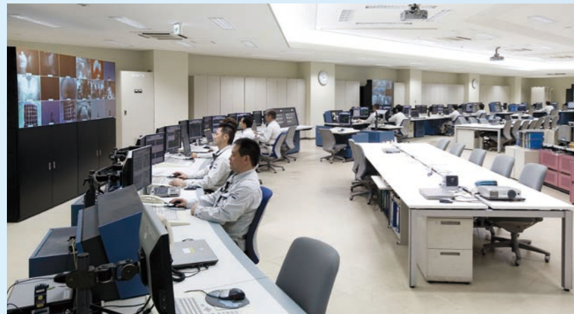
Integrated control room
