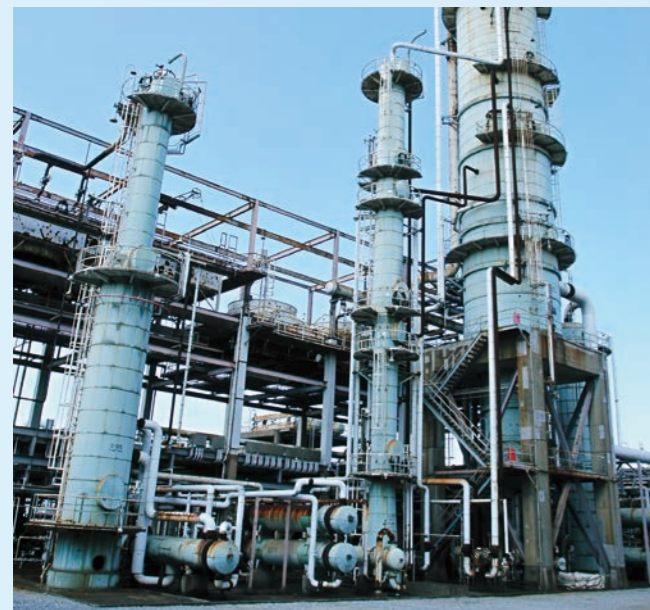
Crude Distillation Unit (CDU)
