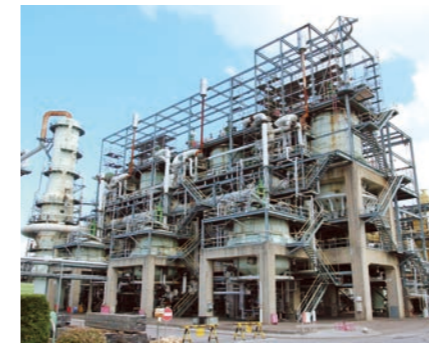
Vacuum residue thermal cracking unit (Eureka Thermal Cracking Unit)
