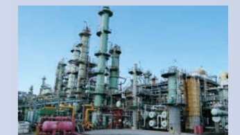
Gasoline Desulfurization Unit
