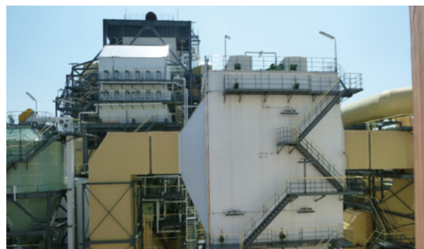
Dry electrostatic precipitator for No. 10 boiler power plant
