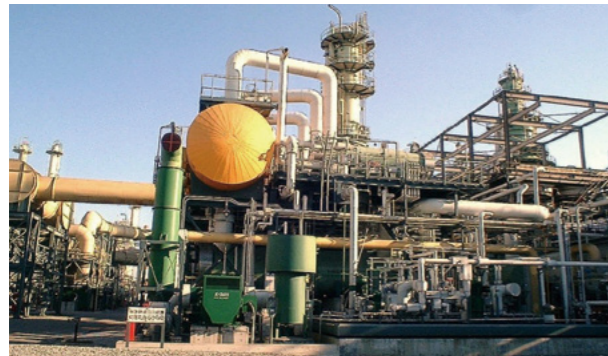
Sulfur recovery equipment
