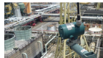
Wireless sensors attached to facilities within the refinery
