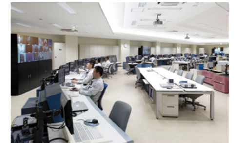
Integrated control room
