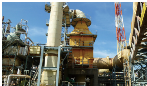
CO boiler flue gas denitrification equipment
