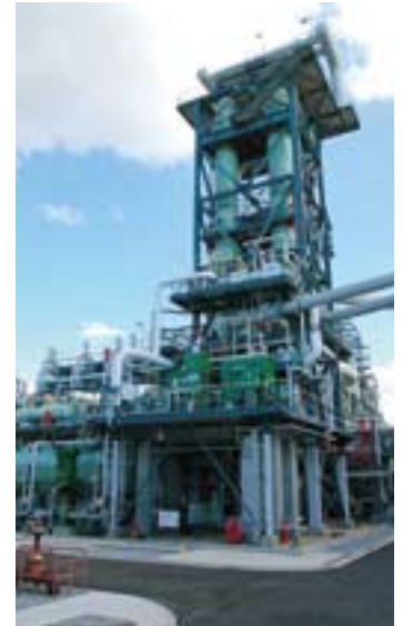
Low-exergy generation system
